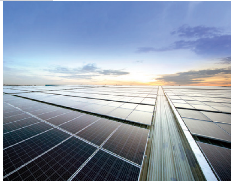
→ Solar panels installed at our Singapore aerospace facilities help fulfil 30% of our electricity needs
